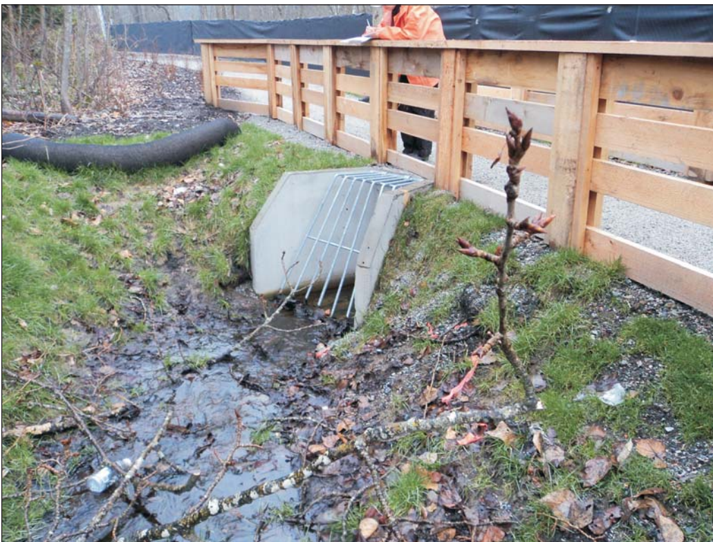
Photograph 12: Culvert on the east end of stream along south boundary of the site.
