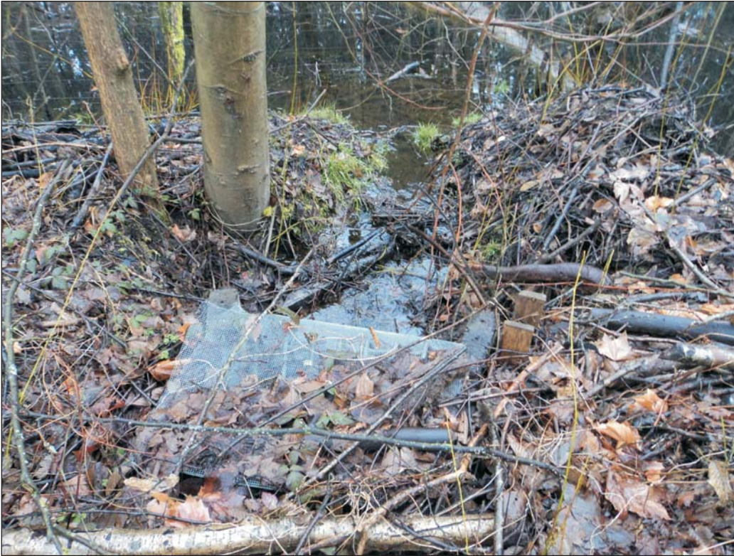
Photograph 11: Culvert on east side of wetland channelling water northeast under University Boulevard.
